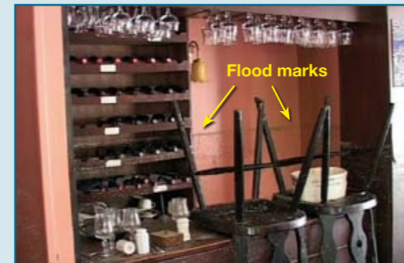
Flood levels can be surveyed from debris marks. Courtesy: Kevin Daly
